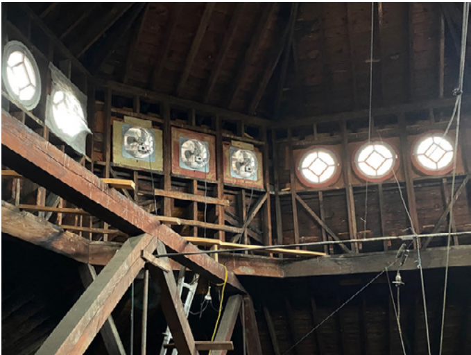
Fans installed in the octagon part of the sanctuary attic
